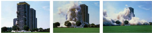
Figure 6.6 Explosives produce large quantities of high-pressure gas. When the gas expands, it does work in demolishing the building
