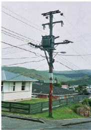
Figure 24.3 Transformers are produced in many shapes and sizes.
