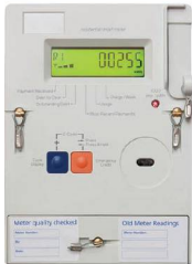
Figure 6.14 A domestic digital electricity meter
